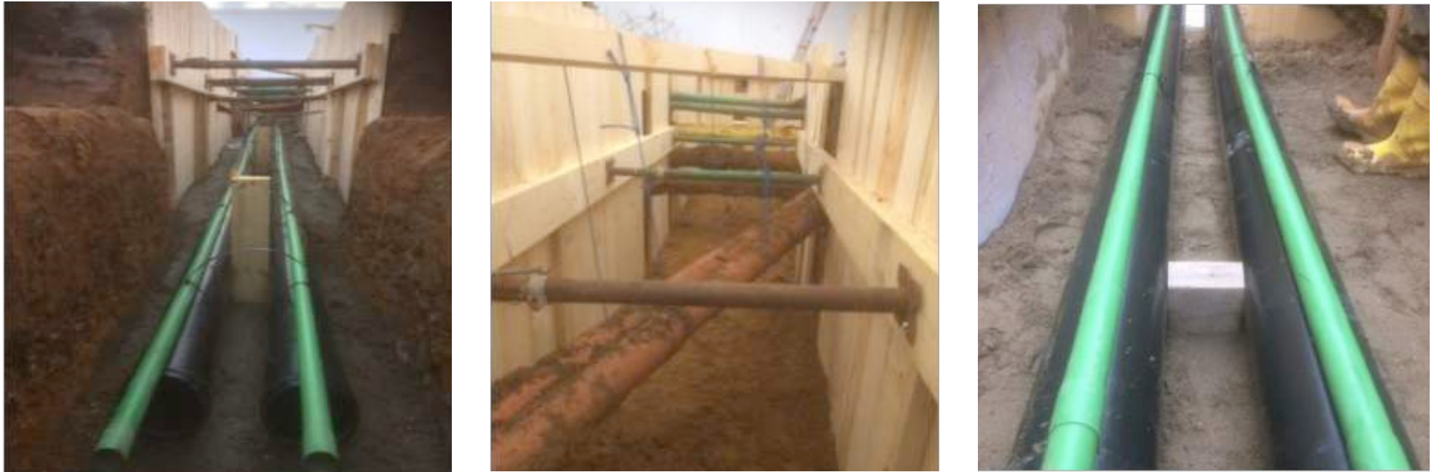
FIGURE 15 TRENCH DUCTS (TIMBERING, CROSSING EXISTING SERVICES, AND AUXILARY CABLE (consent from Prysmian Durkin & Sons).
