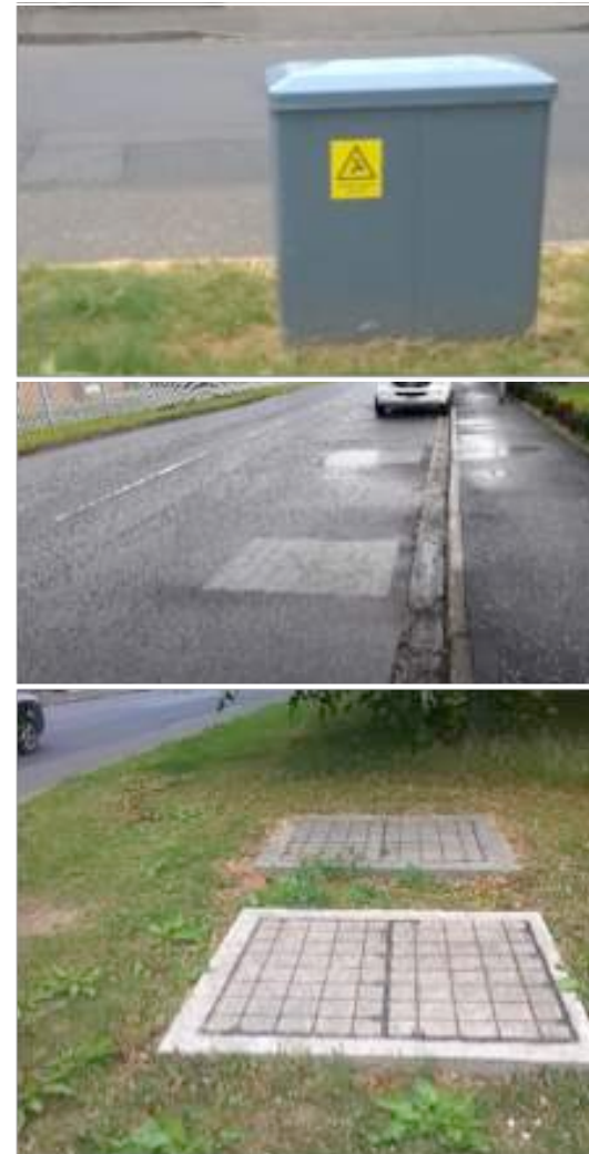
FIGURE 17 EXAMPLES OF JOINT BAY WITH LINK BOXES/PILLARS AND CABINETS (Images courtesy of Prysmian).
